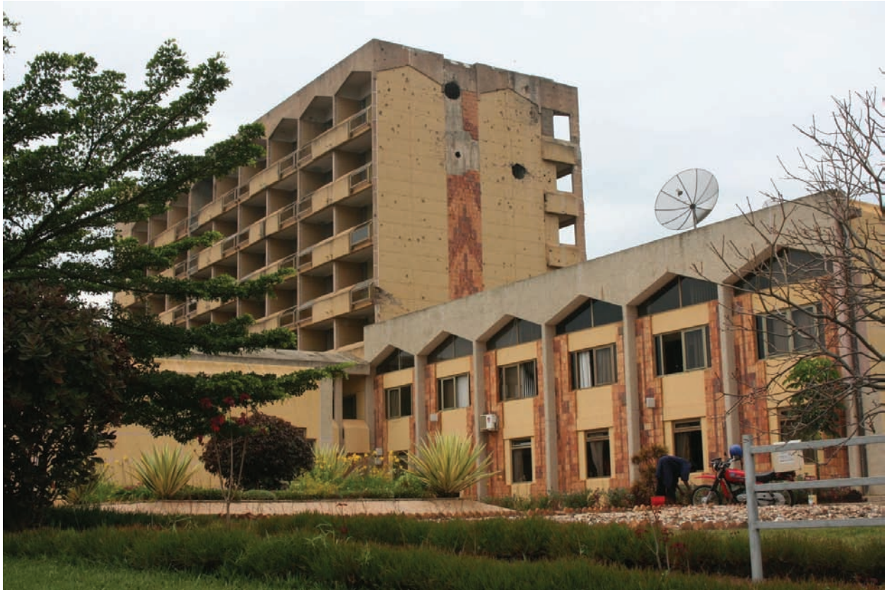
Parliament building, Kigali. Damage to the building from the violence in 1994 is still evident in this 2006 photo. Reconstruction began in 2007. Photo credit: Elizabeth Powley
